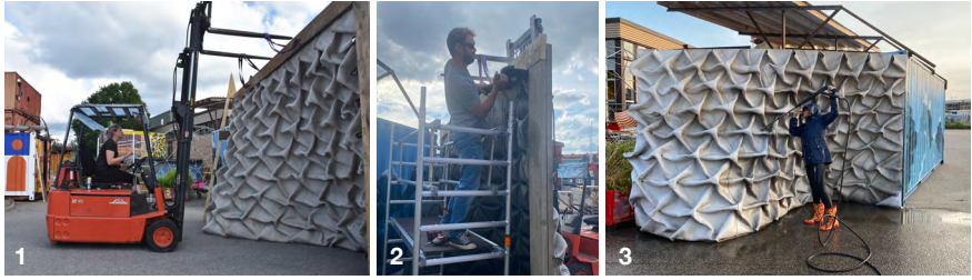
FIGURE 5.61: Wall Three (1) transport and placement, (2) frame removal, and (3) power washing (Source: author).
