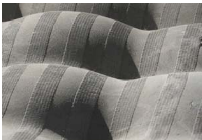
Figure 4: Detail of concrete surface with imprints from the woven fabric pattern of the formwork
